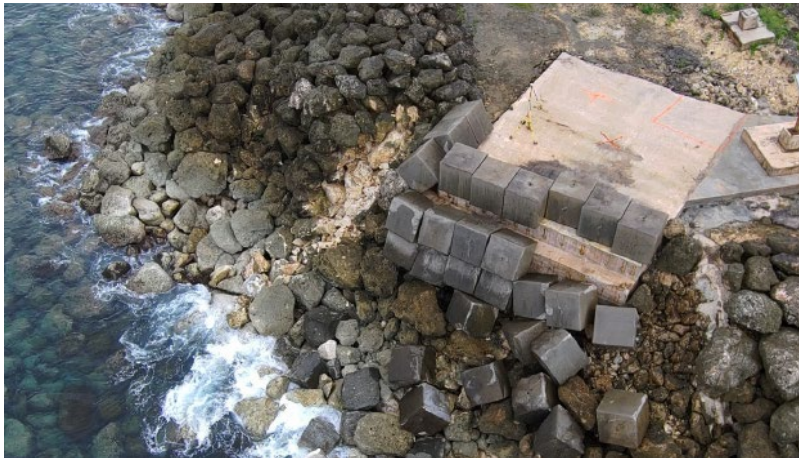
Figure 3-4. Photo of large boulders and concrete blocks falling down the steep incline at the head of the Glass Breakwater armored shoreline.
