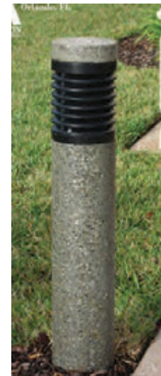
Concrete Bollard Lighting
