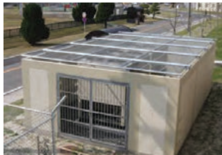
Chainlink enclosure at top of enclosure wall to meet AT/FP requirements
