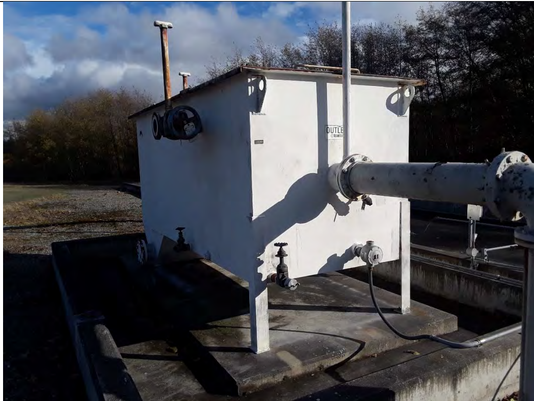
-Aboveground oil/water separator (facing southeast)
