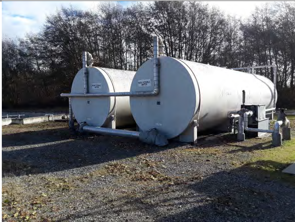
-Water storage tanks (all water used onsite is stored and recycled) (facing southeast)
