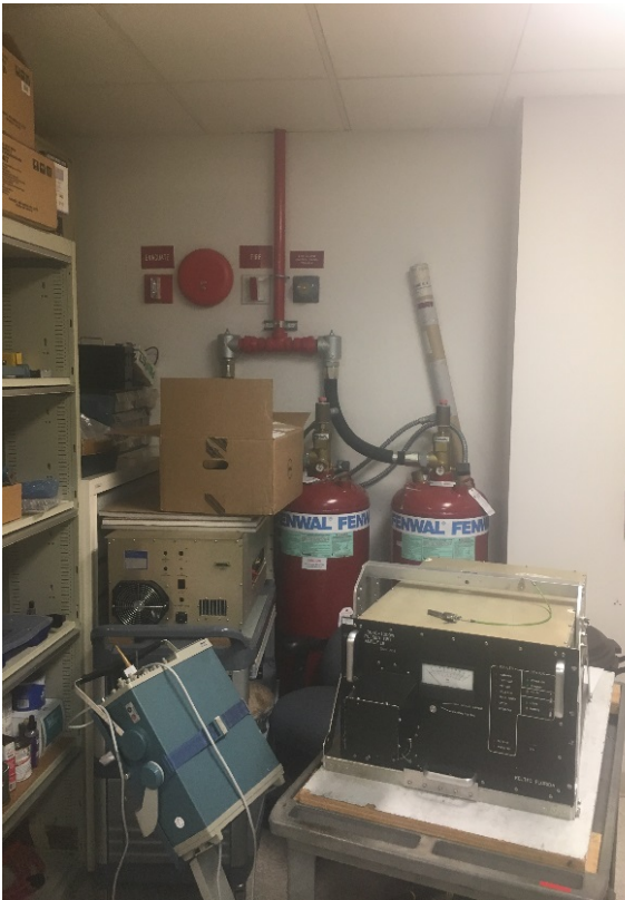
Halon fire suppression system in Building 2807
