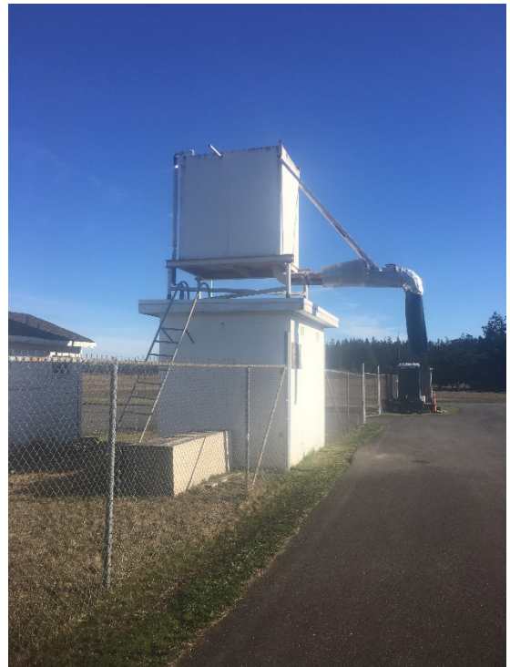
Facility 11 (Potable Water Well Pump House) with PF Tank 11 on roof
