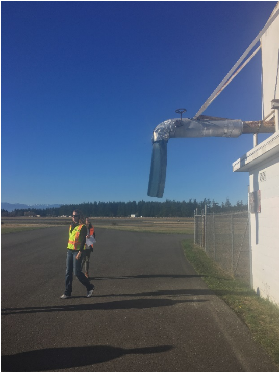
Conduit from FP Tank 11
