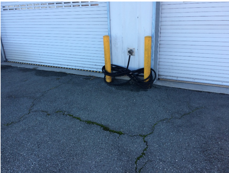
Water spigot and hose on the west-side of Building 2709
