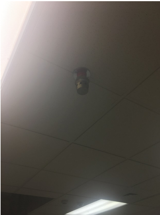
Halon fire suppression system in Building 2807
