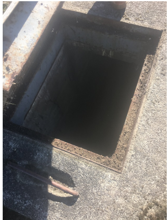
Vault at the north end of the runway next to the optical landing system utility connection
