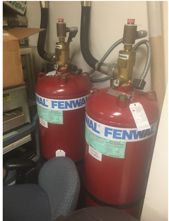
Halon fire suppression system in Building 2807
