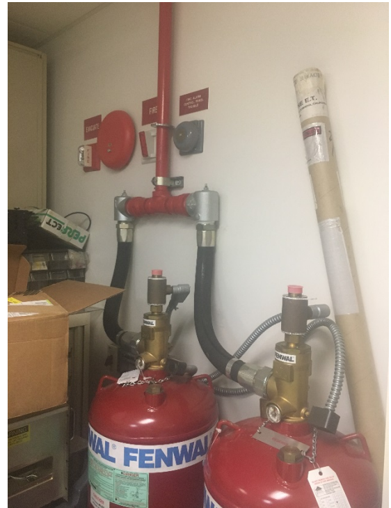
Halon fire suppression system in Building 2807
