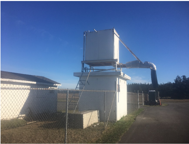
Facility 2 (Airfield Operations Building) (left) and Facility 11 (Potable Water Well Pump House) with PF Tank 11 on roof (right)
