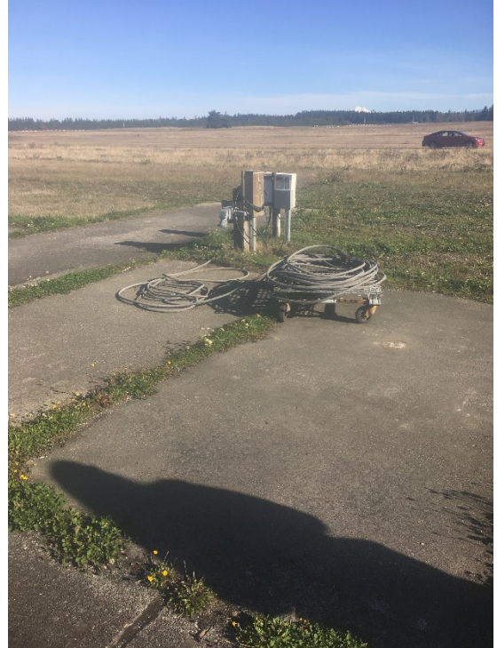
Optical landing system utility connection, north end of runway
