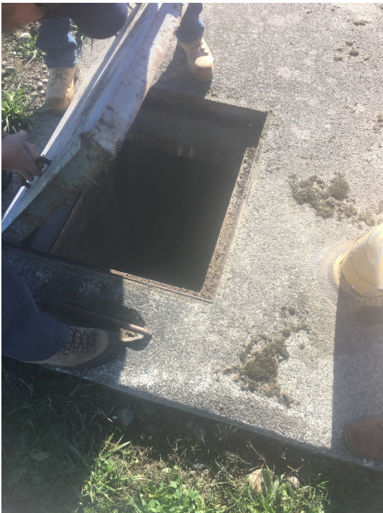
Vault at the north end of the runway next to the optical landing system utility connection
