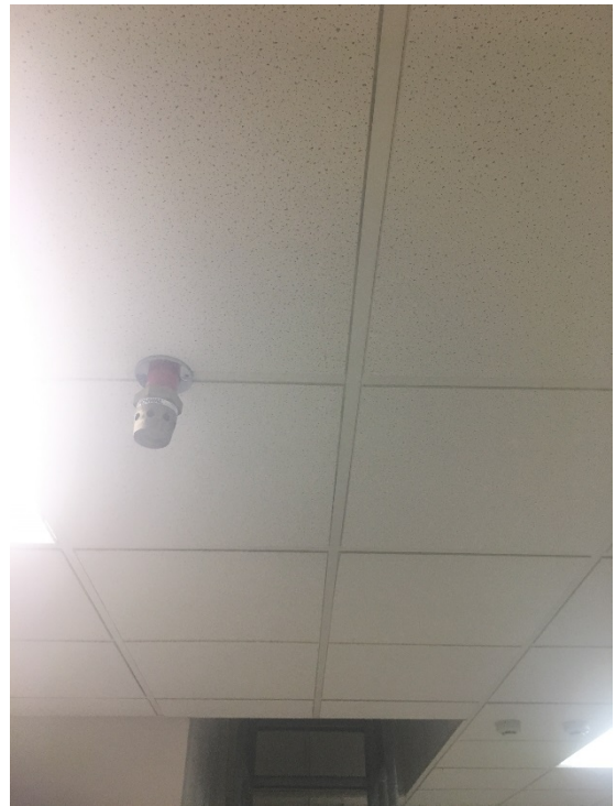
Halon fire suppression system in Building 2807
