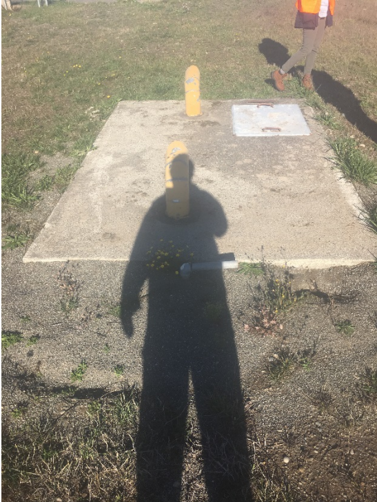
Vault at the north end of the runway next to the optical landing system utility connection
